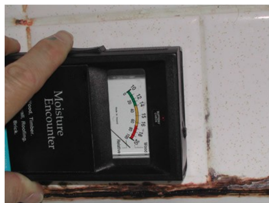
Figure 4: Moisture meter showing damp baseboards
