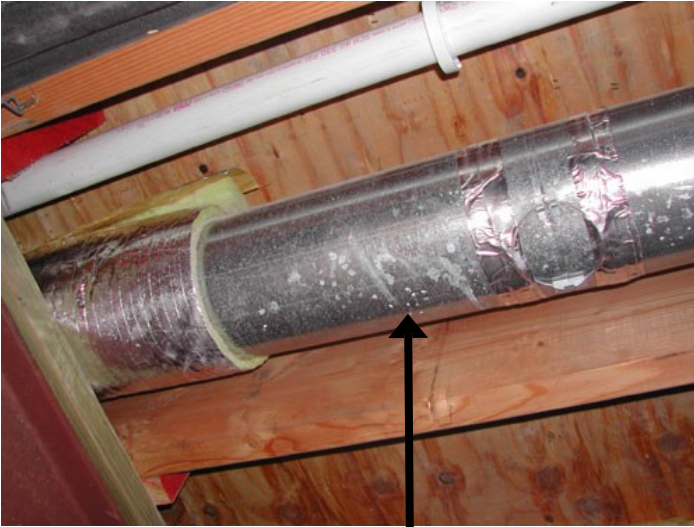
Figure 3: Condensation on pipes
