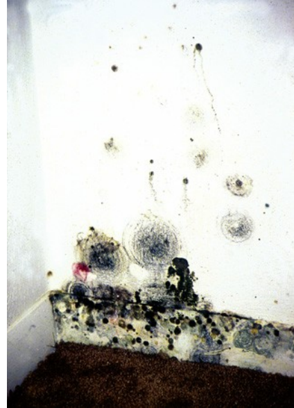
Figure 1: Mold growing on baseboards of a home
