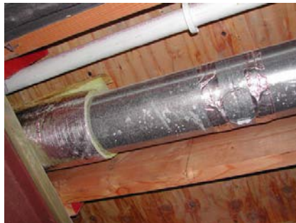
Condensation on pipes
