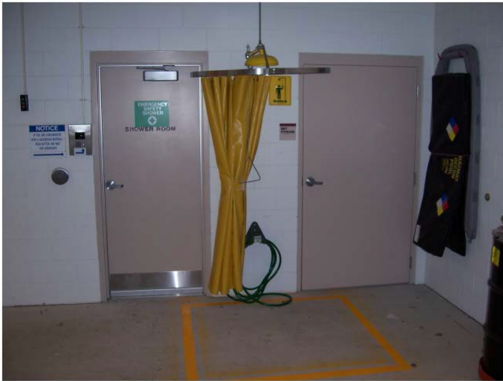
Stationary shower in health care facility
