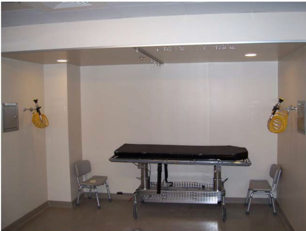
Plumbed line in Emergency room area
